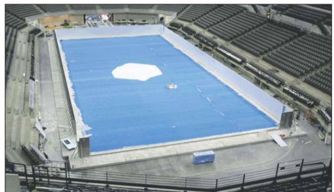
WEDNESDAY, MAY 21: The walls go up and the blue vinyl matting is laid. The side walls came in prefabricated 6.5-foot-wide segments.
