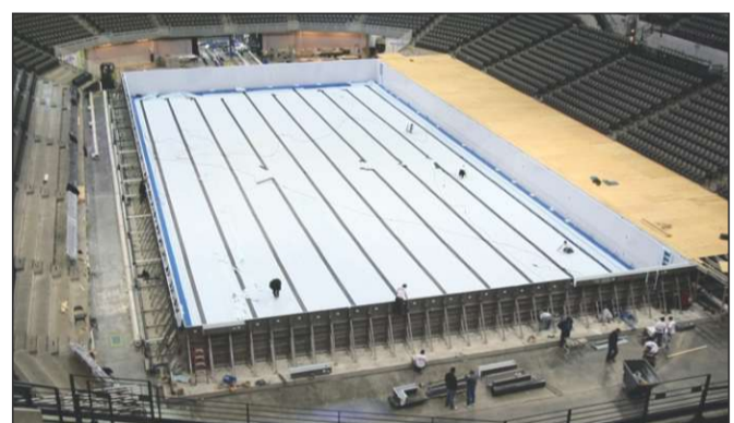
WEDNESDAY, MAY 28: With the vinyl liner down, workers follow with the lanes. Also, at right, is the first scaffolding and plywood for the pool deck.
