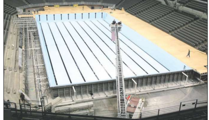
THURSDAY, MAY 29: Omaha firefighters deliver the first 6 inches of water. After allowing the liner to stretch, they finish Friday.
